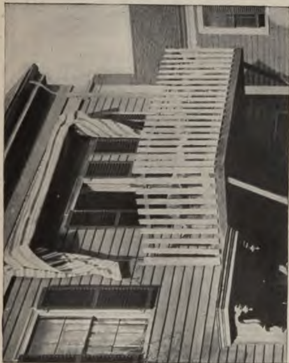
A cheap temporary porch protected by an awning and supported by braces set at an angle
